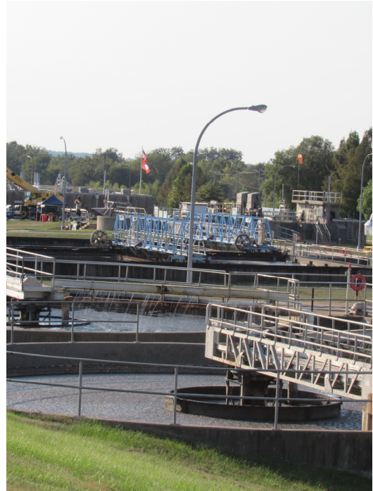
Fourche Creek Wastewater Treatment Facility, Little Rock, AR
