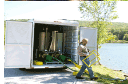
The SDOX™ units can deliver oxygen up to a rate of 3300 lb/day. This system was used in a shallow stream.
