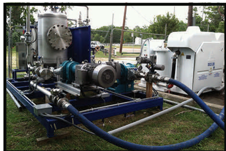
BlueInGreen's SDOX unit in a Houston neighborhood
